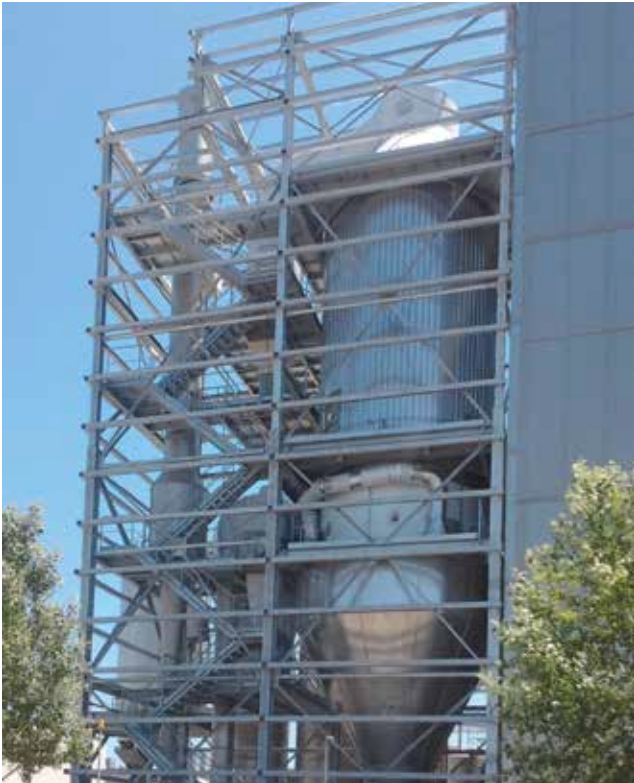
● SPRAY DRYER ITALY, 2011
