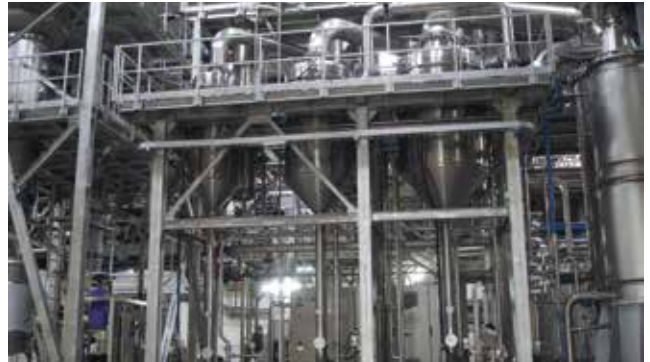
● COMPLETE INSTANT COFFEE PLANT INDONESIA, 2008
