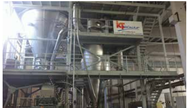
● SPRAY DRYER ITALY, 2014
